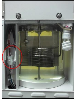
Figure 7. Wiring Disconnection Point
