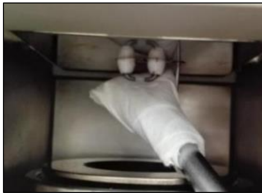
Figure 4: Cleaning Ignition Pins
